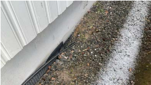
Noe manglende topplist.
