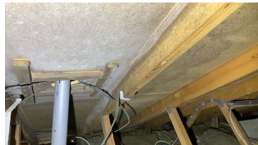
Noe mugg i undertak
