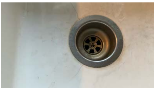
Krakelering i vask.
