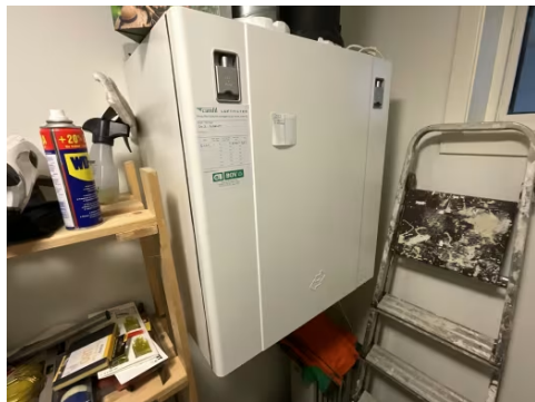
Aggregat i bod.
