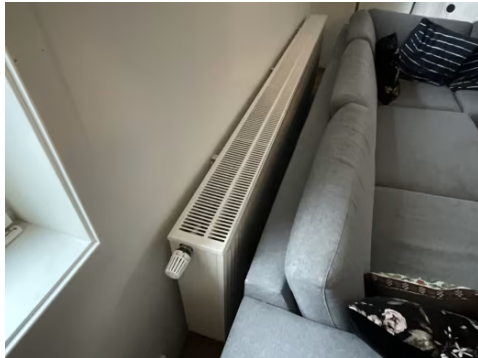
Radiator i stue.
