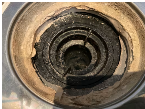
Manglende membran under klemring.
