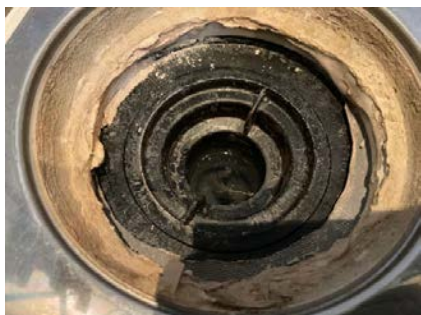
Manglende membran under klemring.
