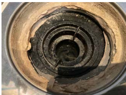
Manglende membran under klemring.
