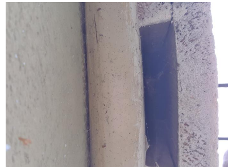
Det mangler Lusing/muse tetting.
