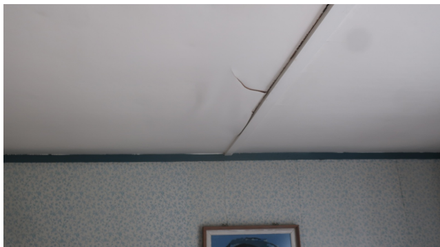
Skade i himling.
