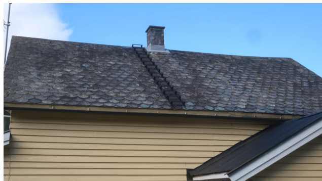
Montert takstige. Noe mosegrodd skifer.
