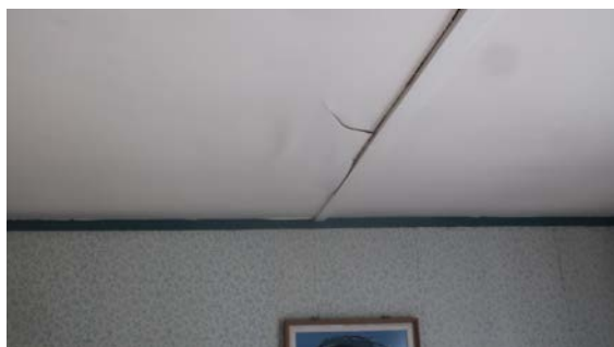
Skade i himling.
