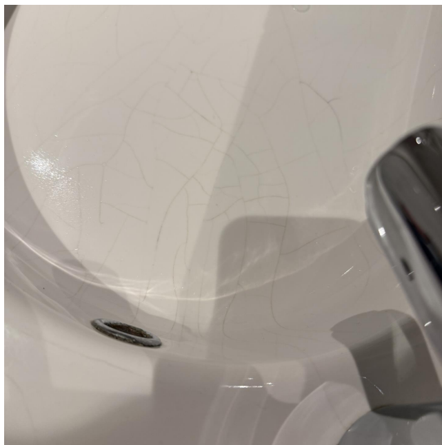
Riss i vask
