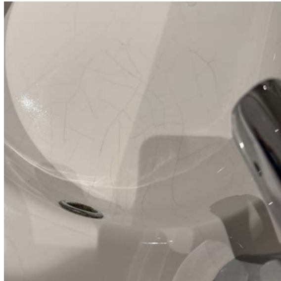
Riss i vask
