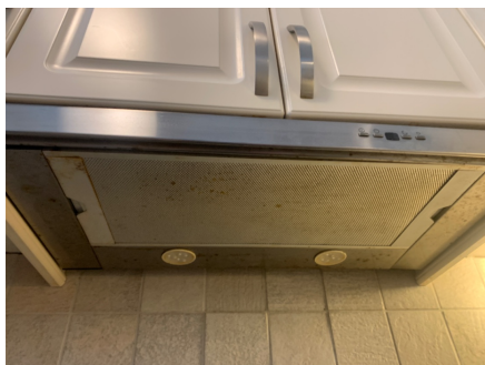
Ventilator over kokesone
