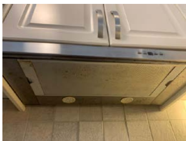
Ventilator over kokesone
