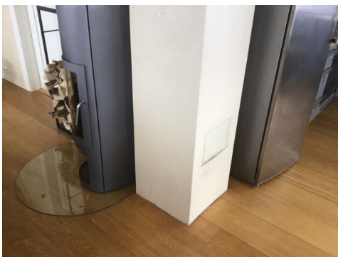
Mangler ildfast plate under feierluke
