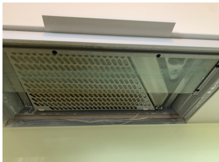
Spjellventilator over kokesonen
