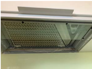
Spjellventilator over kokesonen
