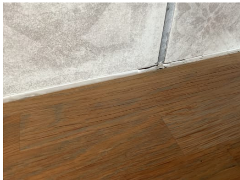
Sprekker i fug.
