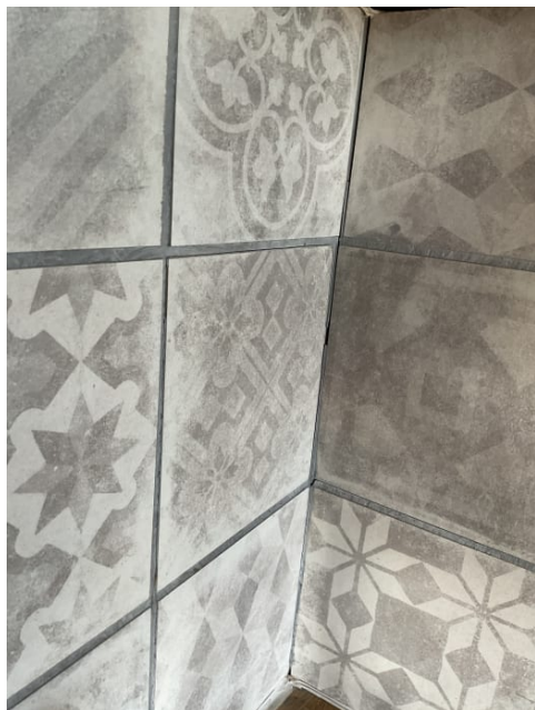
Sprekker i fug.
