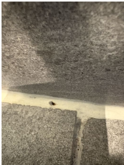
Sprekker i fugemase/silikon
