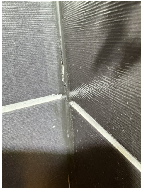
Sprekker i fugemase/silikon
