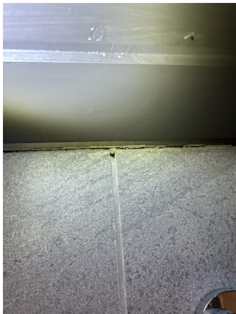
Sprekker i fugemase/silikon
