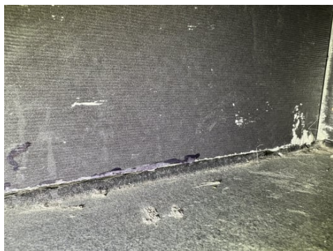
Sprekker i fugemase/silikon
