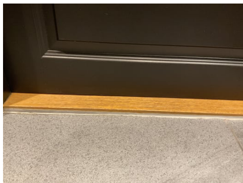
Manglende tilluft bad.
