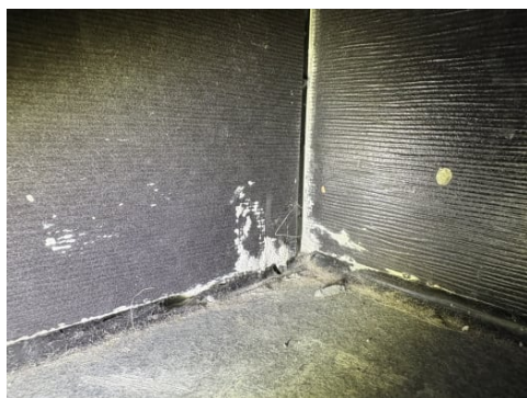
Sprekker i fugemase/silikon
