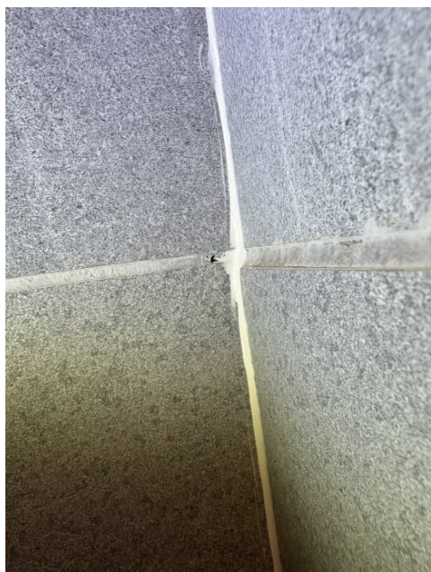
Sprekker i fugemase/silikon
