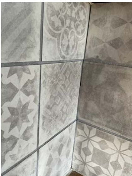
Sprekker i fug.
