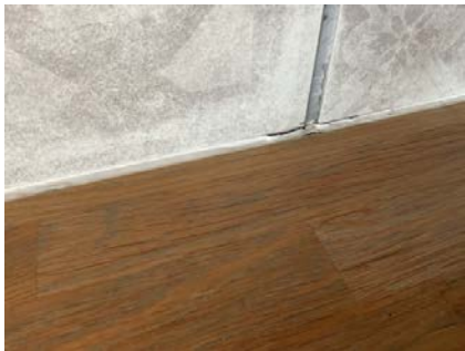
Sprekker i fug.
