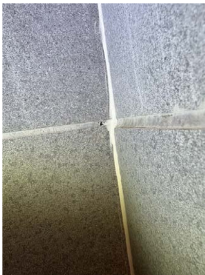
Sprekker i fugemase/silikon
