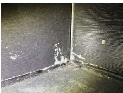
Sprekker i fugemase/silikon
