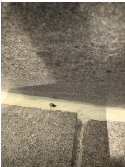
Sprekker i fugemase/silikon
