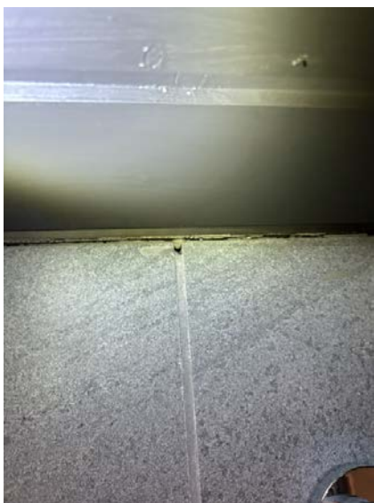
Sprekker i fugemase/silikon
