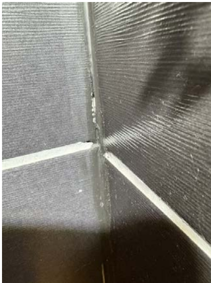
Sprekker i fugemase/silikon
