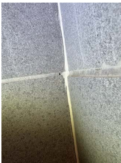
Sprekker i fugemase/silikon
