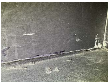
Sprekker i fugemase/silikon
