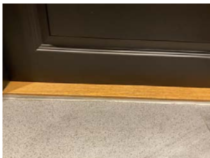
Manglende tilluft bad.
