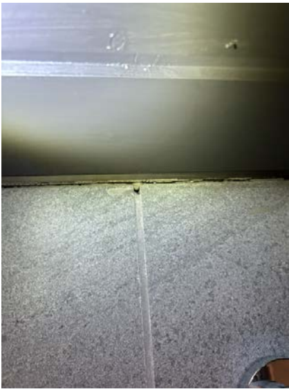
Sprekker i fugemase/silikon
