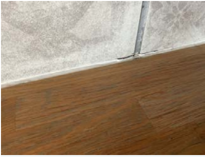
Sprekker i fug.
