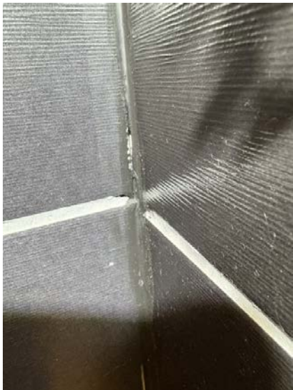
Sprekker i fugemase/silikon
