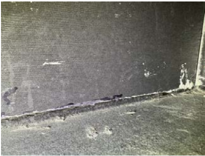
Sprekker i fugemase/silikon
