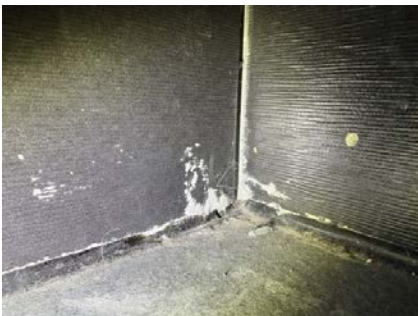
Sprekker i fugemase/silikon
