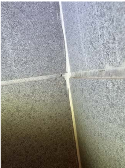
Sprekker i fugemase/silikon
