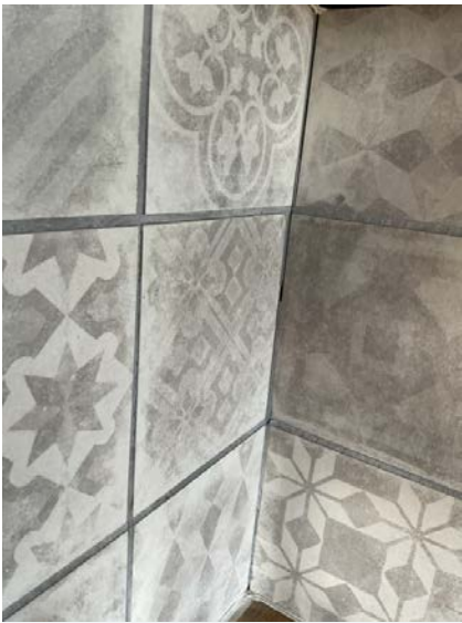
Sprekker i fug.
