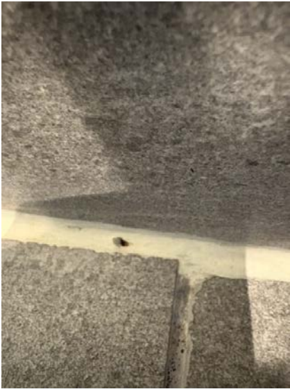
Sprekker i fugemase/silikon
