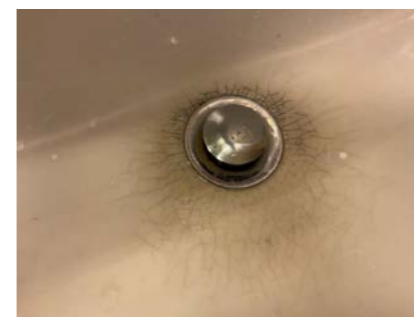
Riss/sprekker i servant.
