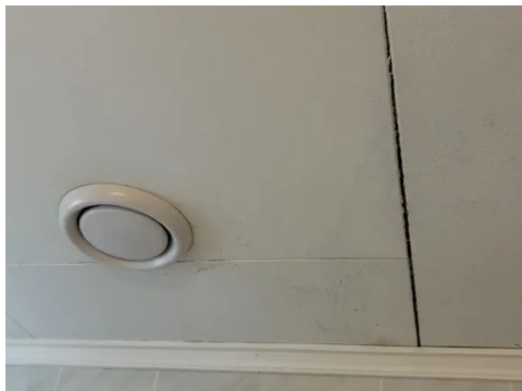
Kondensmerker i himling.
