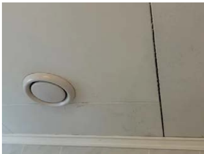
Kondensmerker i himling.
