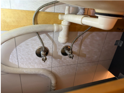
Røropplegg under servant.
