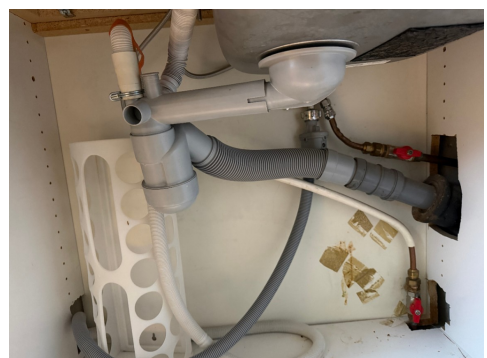
Røropplegg under vask.
