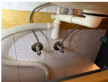
Røropplegg under servant.
