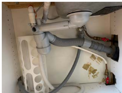
Røropplegg under vask.
