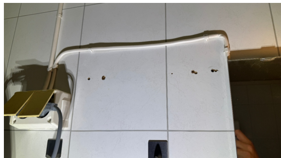
Skruehull i veggplater.
