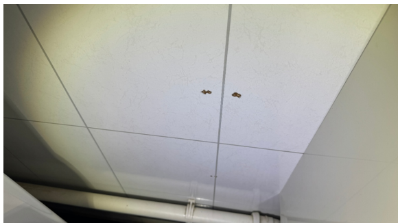
Skruehull i veggplater.
