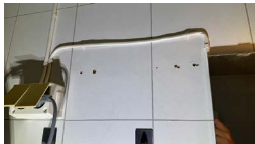
Skruehull i veggplater.
