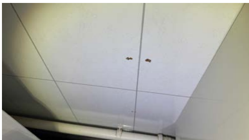
Skruehull i veggplater.
