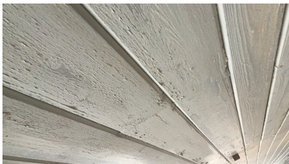
Slitasje i himling.
