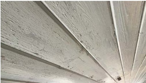
Slitasje i himling.
