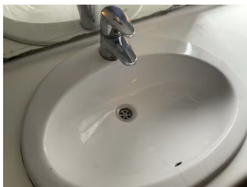
Riss i servant.
