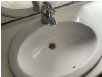
Riss i servant.
