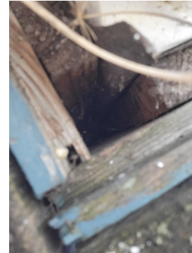
Manglende museband under kledning.
