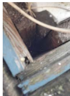
Manglende museband under kledning.
