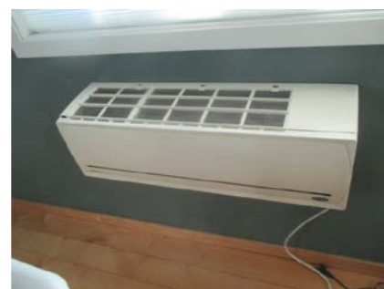
Noe eldre varmepumpe i stue.
