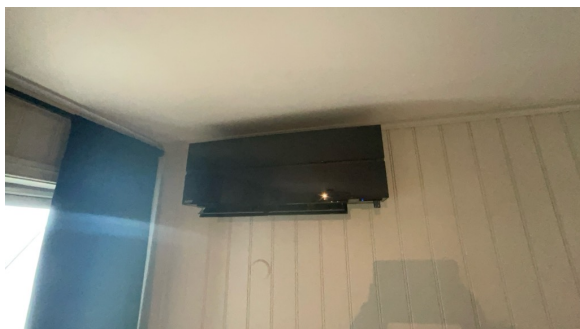
Varmepumpe, innvendig aggregat.
