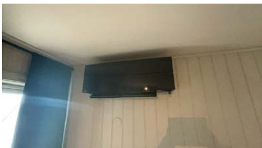
Varmepumpe, innvendig aggregat.
