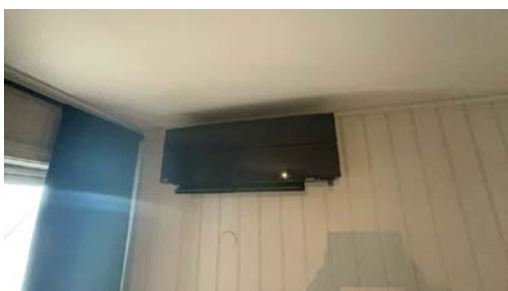
Varmepumpe, innvendig aggregat.
