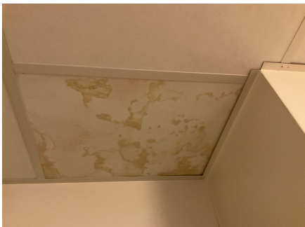
Eldre fuktskade i himlingsplate
