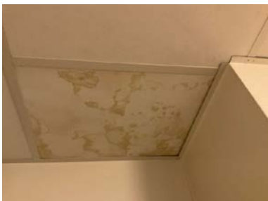
Eldre fuktskade i himlingsplate
