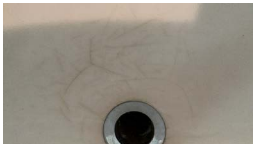
Riss i vask.
