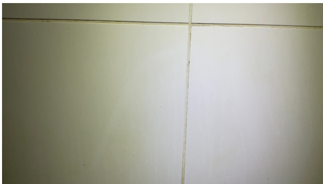
Riss i fuger.
