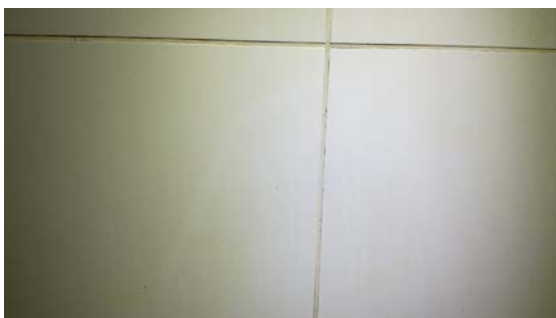
Riss i fuger.
