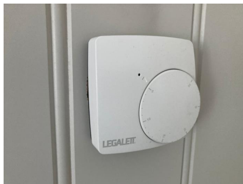
Termostater for gulvvarme.
