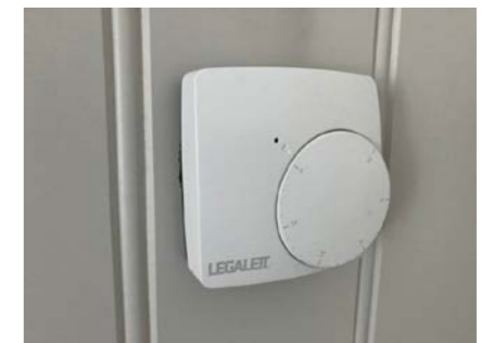
Termostater for gulvvarme.
