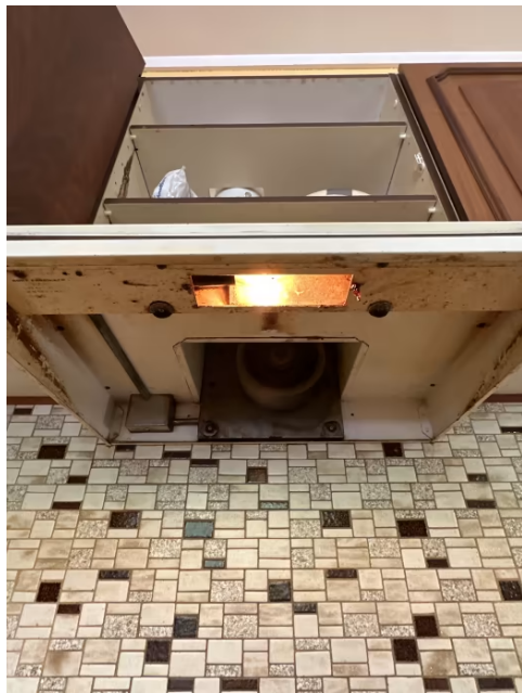
Vifte mangler filter.
