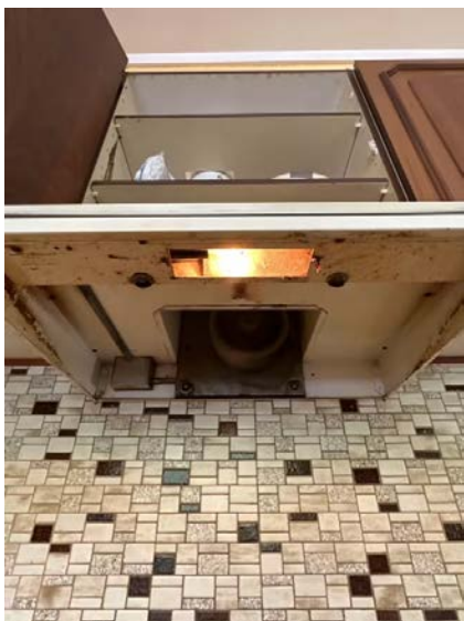
Vifte mangler filter.
