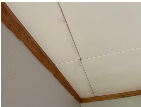
Skader i himling.
