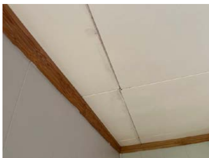
Skader i himling.
