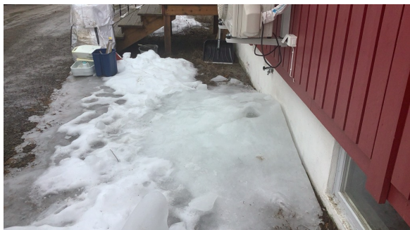
Isdannelse under varmepumpe.
