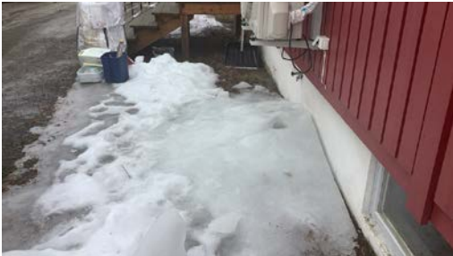
Isdannelse under varmepumpe.
