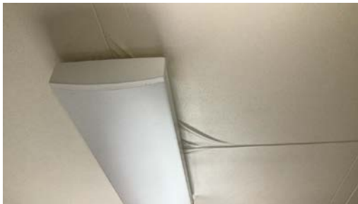
Folieslipp i himling.
