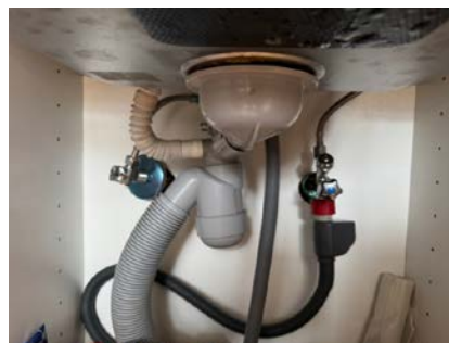
Røropplegg under vask.
